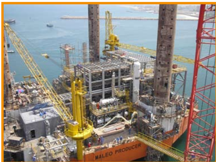
The upgrade and topsides installation of Maleo MOPU Producer took place at a conversion yard in Sharjah, UAE
